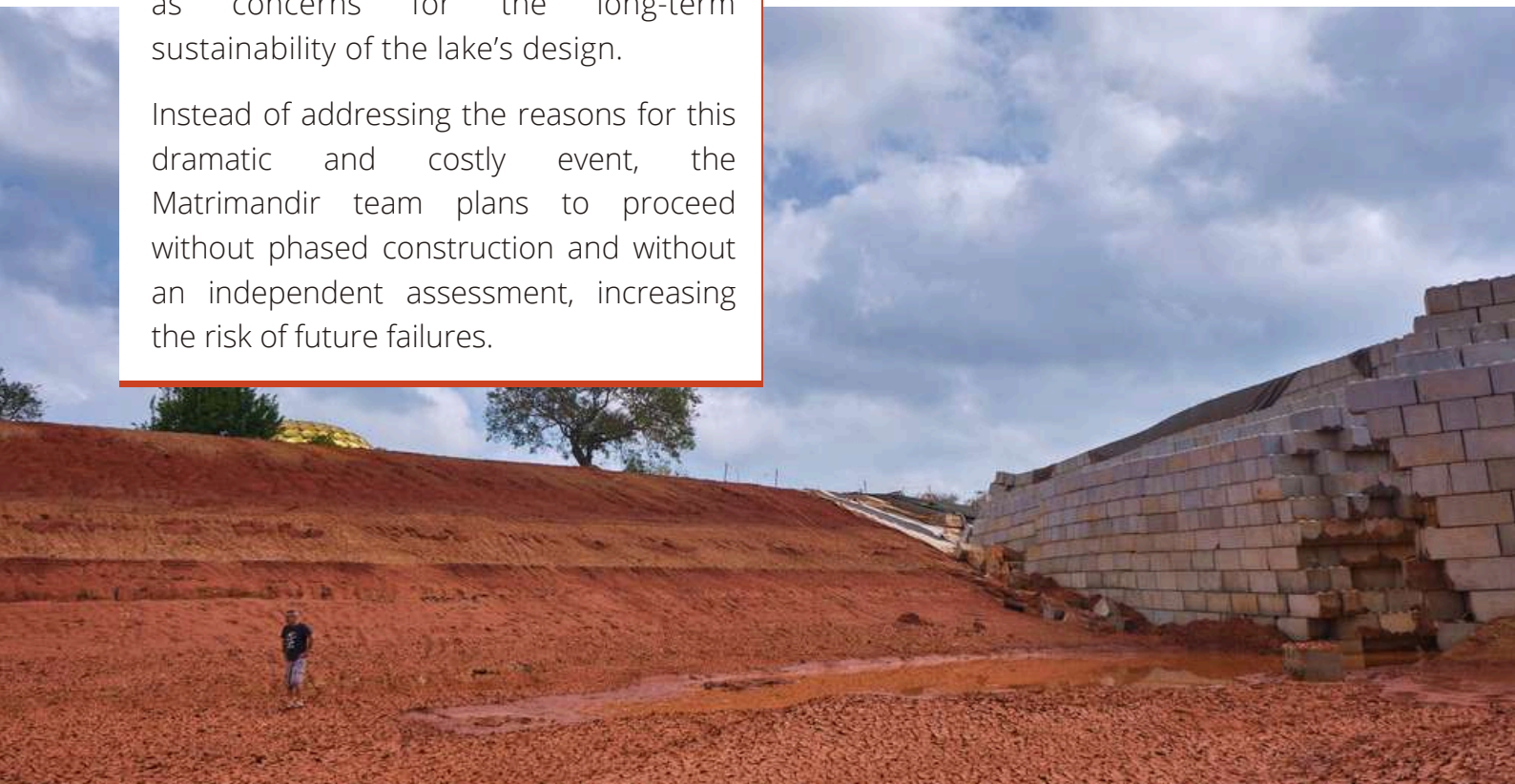
Matrimandir lake heavily damaged by Cyclone Fengal, December 2024
