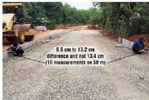
Fig. 29: Never the proper slope: 1.26% to 1.97% and not 2%
