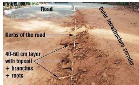
Fig. 6: Roots and branches below the kerbs of the road
