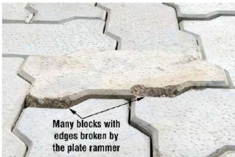
Fig. 18: Broken edges caused by the plate rammer
