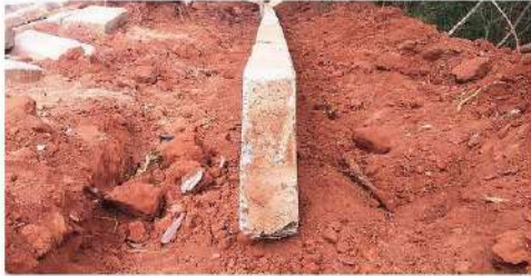
Fig. 20: Kerbs are laid on the soil and not on cement mortar
