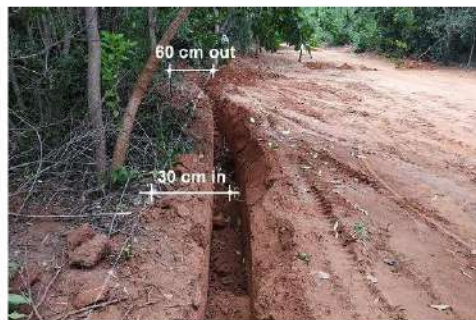
Fig. 36: Totally inaccurate location of the HT cable
