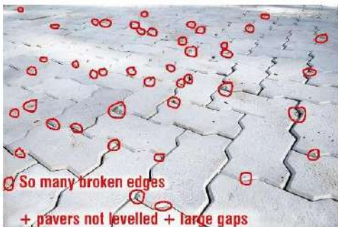
Fig. 14: Unevenness of the surface & broken edges
