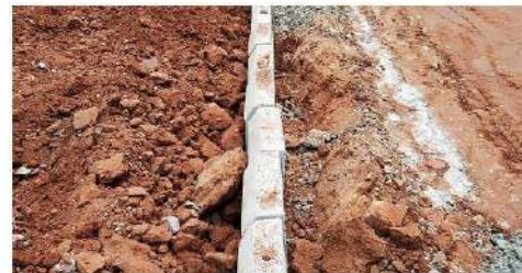
Fig. 23: Kerbs are not aligned properly and move
