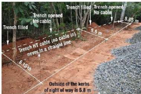
Fig. 38: Trench never in a straight line with no cable inside
