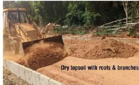
Fig. 2: Dry topsoil which cannot be compressed
