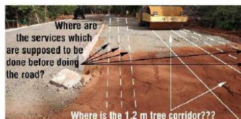
Fig. 6: No provision for services and for the tree corridor
