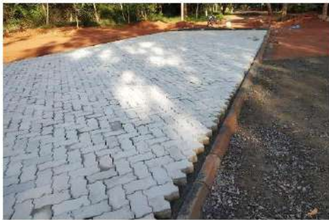
Fig. 42: Pavers laid very badly
