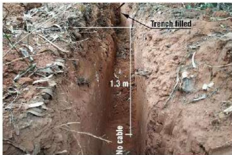
Fig. 40: Trench 1.3 m deep with no cable inside
