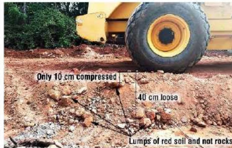
Fig. 15: 45 cm of loose red soil = not well compressed
