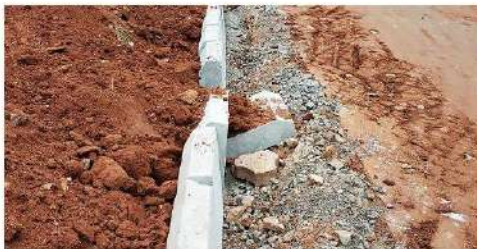
Fig. 22: Kerbs are falling and moving a lot
