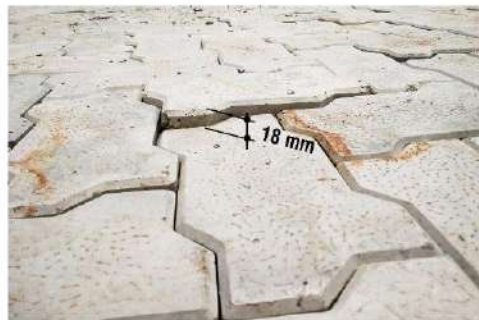
Fig. 19: Quality of levelling pavers = 18 mm difference here
