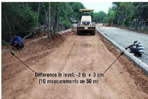
Fig. 30: Difference of levels between road and right of way
