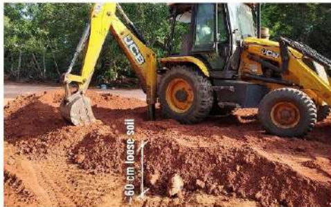
Fig. 16: 60 cm of loose red soil at once = far too thick
