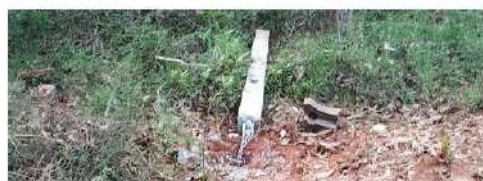
Fig. 4: One of the broken poles, installed by PKS
