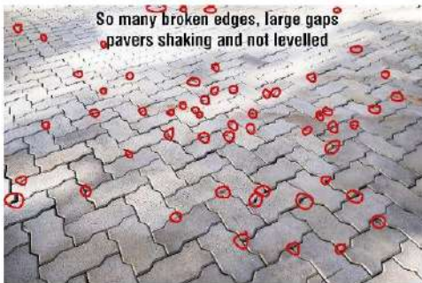
Fig. 12: So many pavers damaged, shaking and not levelled
