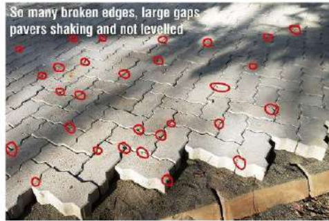
Fig. 11: Surface once rammed = blocks shaking & broken
