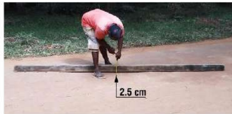
Fig. 66: Existing road at Gaia: deformation over 3.6 m
