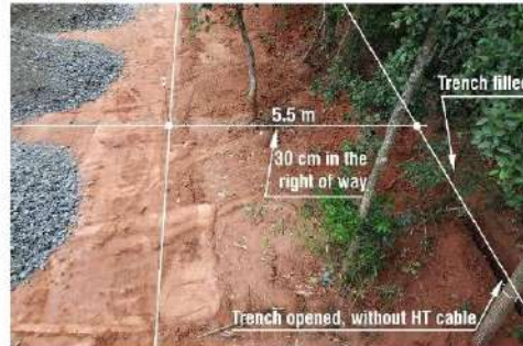
Fig. 37: Trench 30 cm inside and no cable
