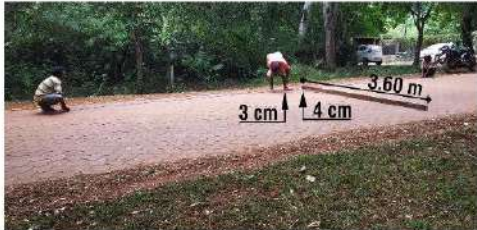
Fig. 67: Existing road at Arka: the most damaged part
