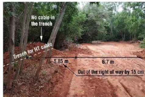
Fig. 39: Trench 15 cm outside and no cable
