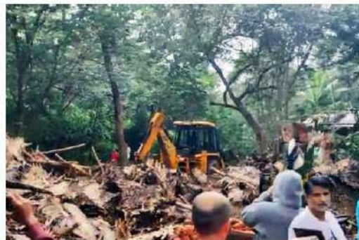
Fig. 12: Savage destruction without notice
